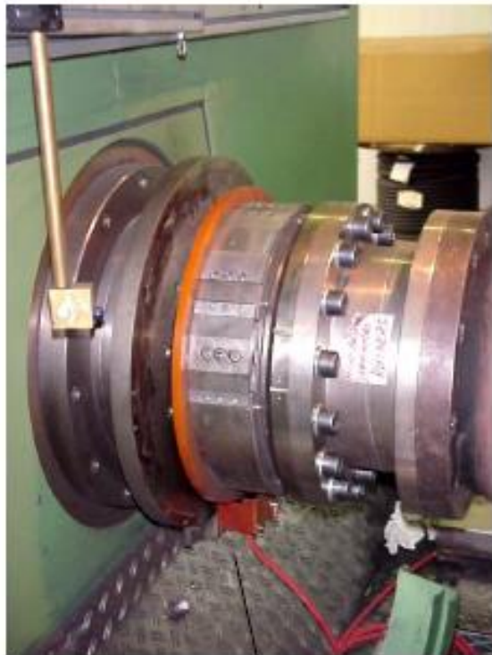
Stator Coil/Antenna Pickup
